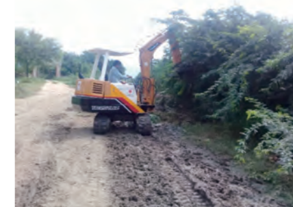
A backhoe that is doing a great job in repairing roads in Tha Pyay Thar Village [Grant from the Government of Japan]
